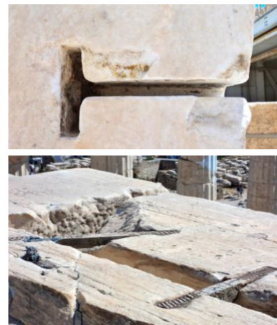
Figure 12: Oxidized marble members and iron clamps
