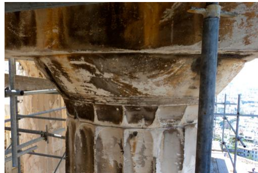
Figure 10: Soot buildup on marble surfaces from carbon monoxide
