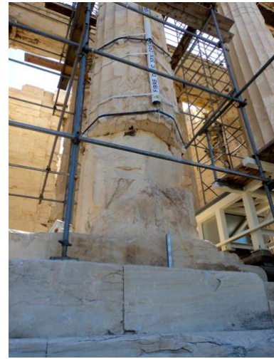
Figure 11: An accelerograph attached to a shifted column
